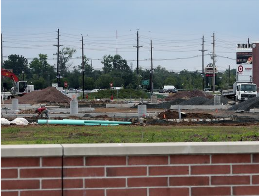
A new transit oriented village , Main Street North Brunswick, is being constructed in the township at 2300 Route 1 North. Also Pulte Homes is building the new town homes The Heights at Main Street at the site. Both are photographed on Tuesday August 2, 2016. (Photo: Mark R. Sullivan/Staff Photo)
